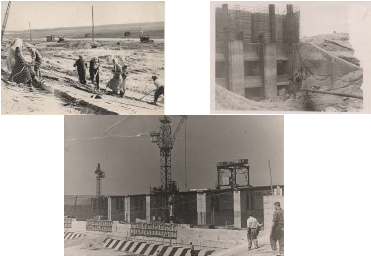
Fig. 3. Archival photos of the construction of the Pechenihy reservoir from the Museum of Local Lore of the Pechenihy district. (Source: T. A. Sulima)
